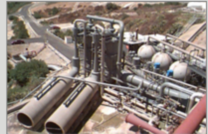
VETS Steam Plant
